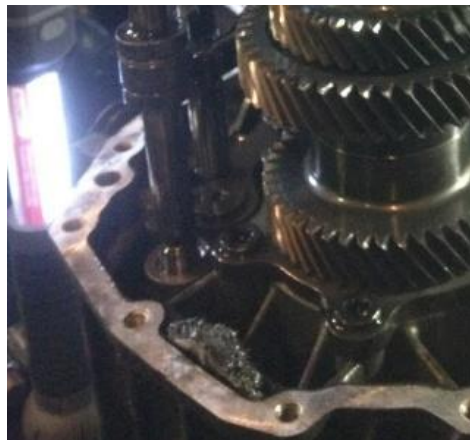
Figure 1: Pinion Bearing Grease Accumulation on Magnet
