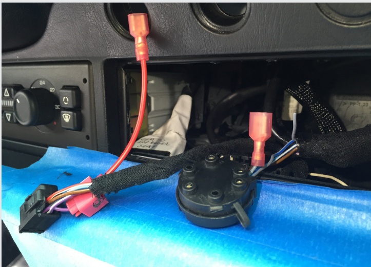
Add connectors Add insulated connectors to solid gray wire coming from fog light switch connector, and to new wire you attached to solid violet wire of rear defroster switch harness.
